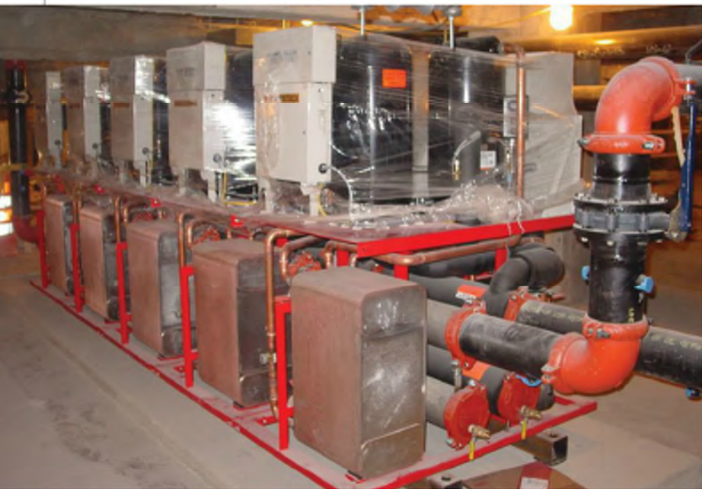
Figure 3: An end view shows five modular chillers and a heat exchanger on the bottom of the units with two compressors on the top. For this project, a modular chiller was the only option for the basement of an existing building due to space limitations.
