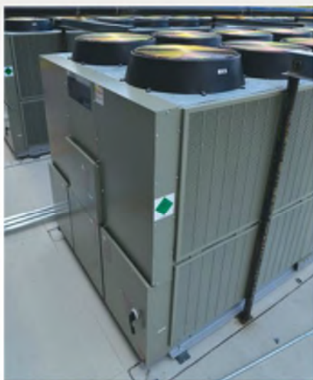
Figure 4: This shows two 400-ton air-cooled screw chillers in parallel for an industrial building.
