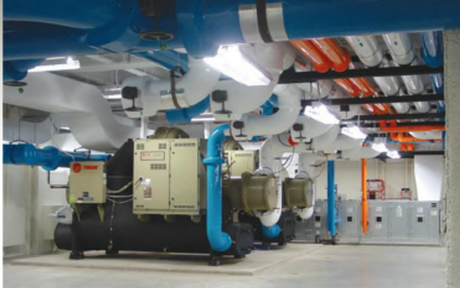
Figure 2: Two 500-ton water-cooled centrifugal chillers serve an office building with space for future chillers.
