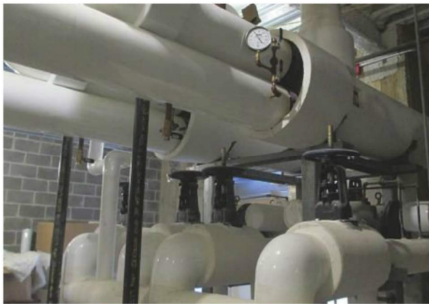
Figure 4: Multiple branch condensate piping discharges into a main condensate pipe with top discharges.
