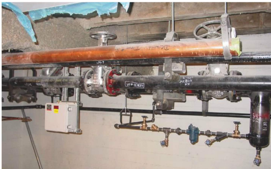
Figure 2: A steam drip leg and trap on a main high-pressure steam pipe upstream of a flow meter are shown.
